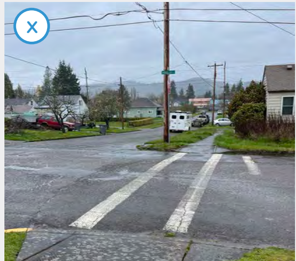
Many crosswalks on local streets in Sheridan use standard stripes, but could be upgraded to high-visibility, continental markings.
