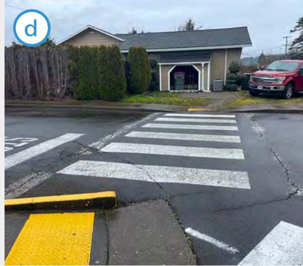
Curb ramps with yellow tactile warning surfaces (in compliance with the ADA) are present at the intersection of Cornwall St and 3rd St, but concrete curbs hinder a smooth transition from roadway to sidewalk.
