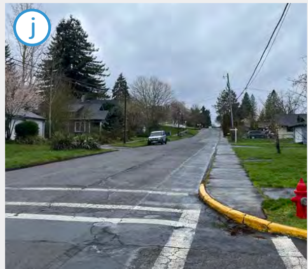
ADA-compliant curb ramps are also missing on the north leg of the intersection of Jefferson St and 1st St. However, the curb ramps on the south leg of the intersection are up to date.
