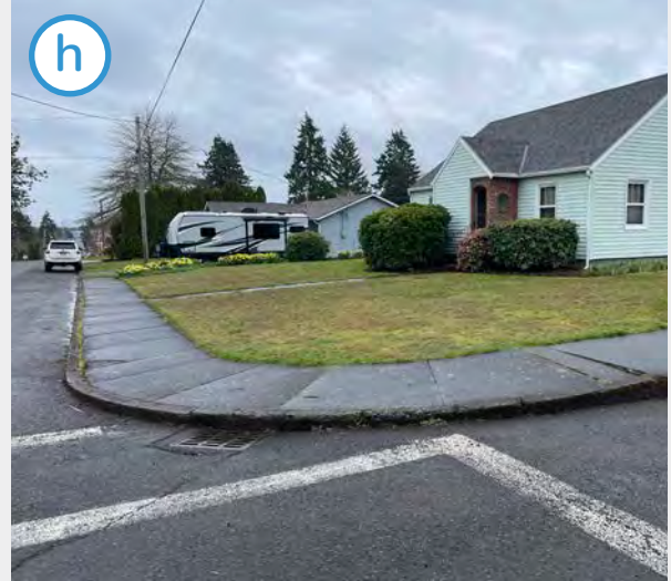
The curbs at the corners at Jefferson St and 3rd St are not ADA compliant.
