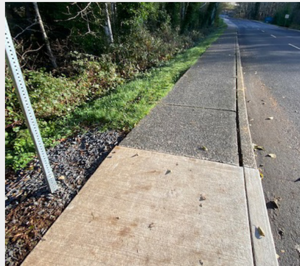
Sidewalks on the north side of Spruce Dr are damaged, uneven, and cracked in certain areas.
