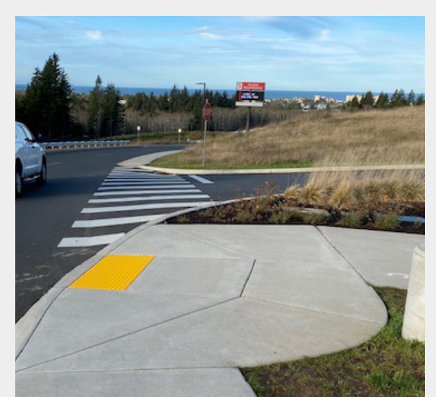
Curb ramps along Spruce Dr, up the hill to the middle/high school. Curb ramps do not align with crosswalks, making it difficult for students to access the crosswalk, especially for people with disabilities.
